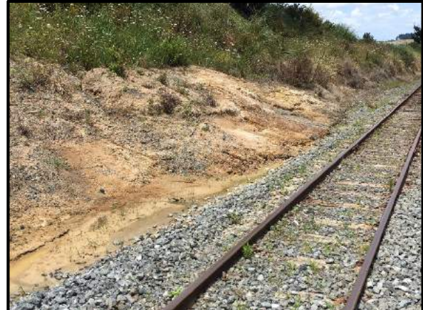
Photo 6: Railroad cut on the west side of the rail road, near the southern end of the study area. Note the water seeping from the cut and the slope failing at less than 1V:3H slope batter.
