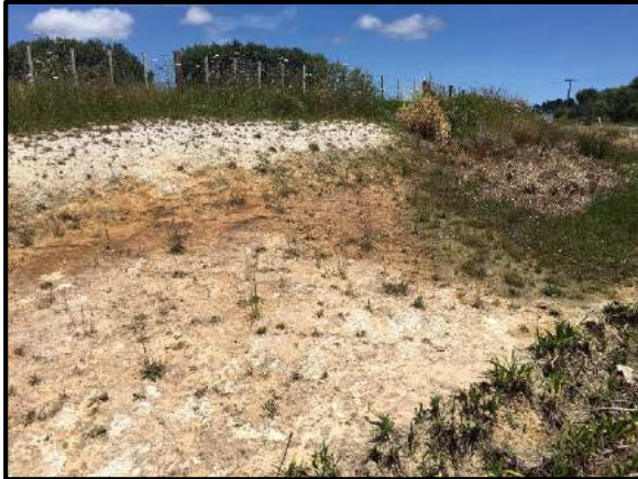
Photo 5: Road cut on the south side of Oneriri Road. Note the water seeping from the shallow cut.
